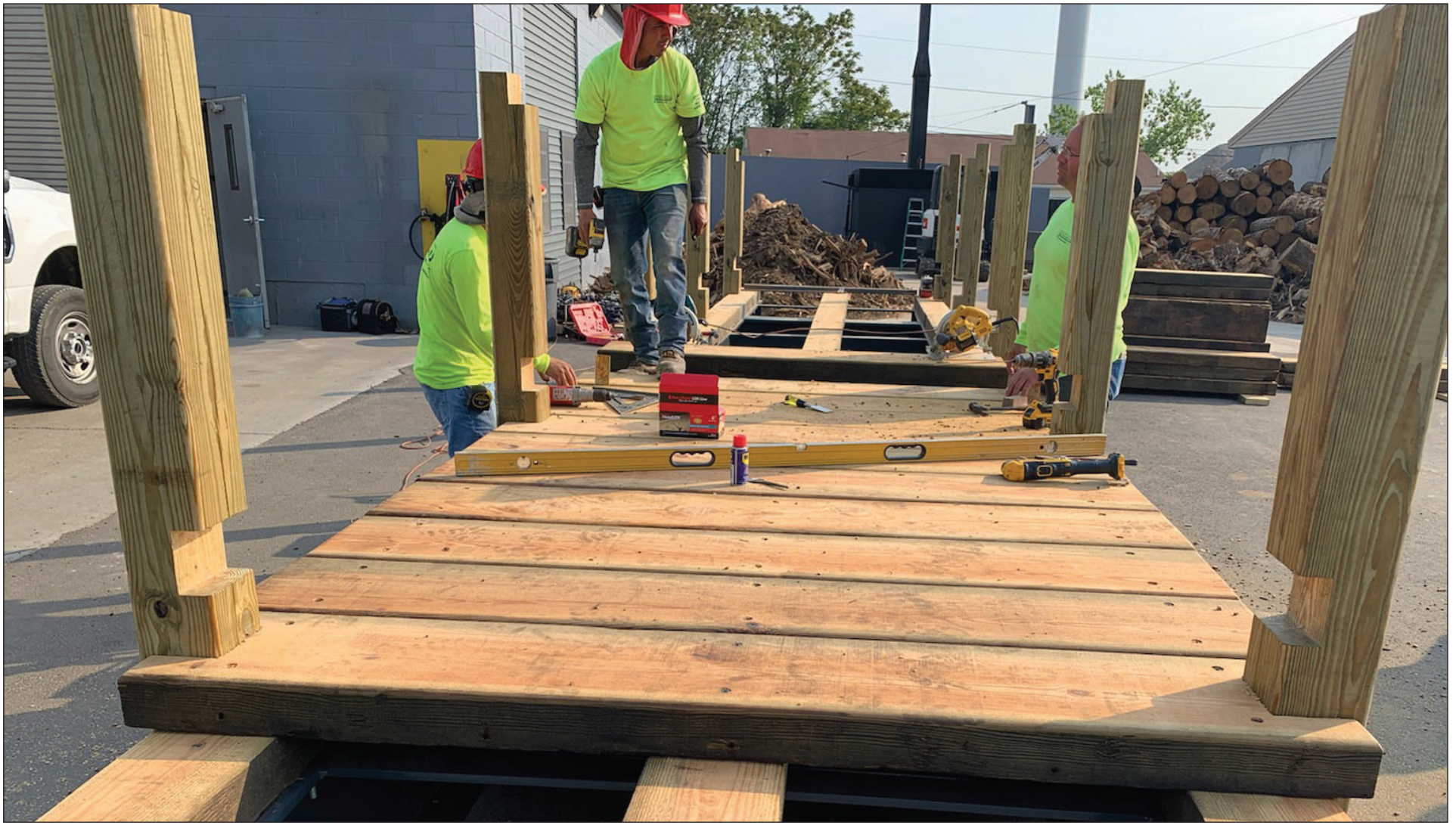
HARD AT WORK: Workers from JR Vinagro Corp., a Johnston construction company, prefabricate a footbridge for Johnston War Memorial Park's walking path. The bridge will be installed next week. (Photo courtesy of Mayor Joseph M. Polisena)
